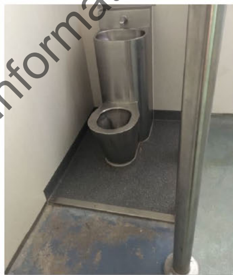
Photo: Toilet in secure unit room
