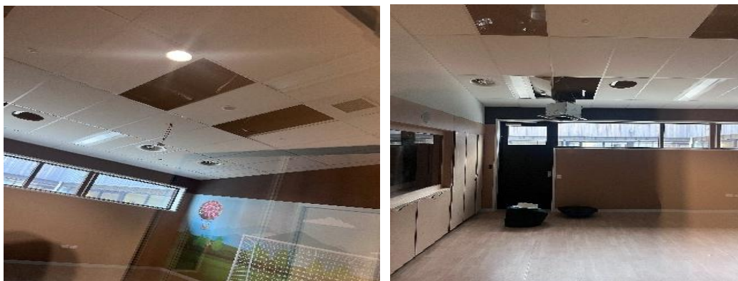
(Broken roof of the inside gym)
