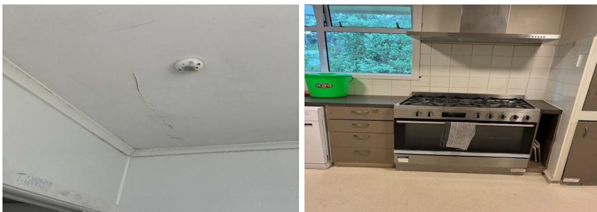
(Left) Paint peeling and tagging, and (Right) current kitchen area
