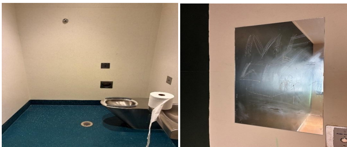
The metal toilet with shower head (left) and the mirror in the bathroom (right)
